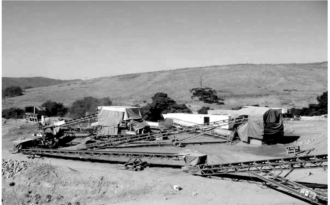
The screening plant in the OB/OD area screened 260,000 cubic yards of soil.
